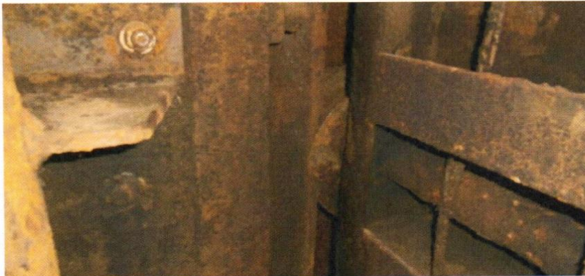
Left: Backside of gate that needs to be replaced
